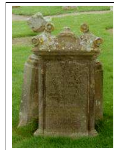
Figure 45 A headstone that has lost its finial
