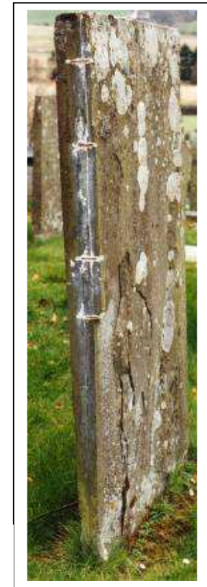
Figure 54 Headstone with iron staples
