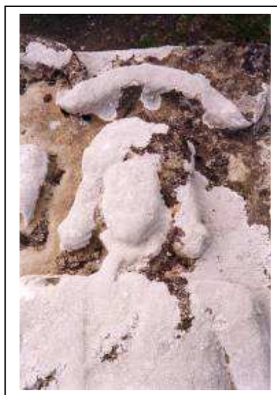
Figure 63 Extent of lichen growth here is major
