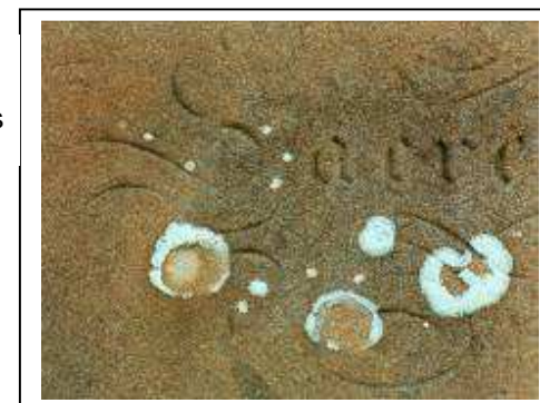
Figure 61 Damage to stonework associated with lichens
