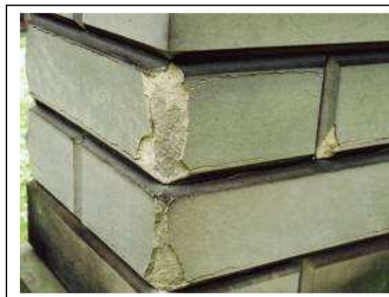
Figure 77 Moderate contour scaling on flat surface
