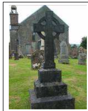
Figure 83 Major pollution staining
