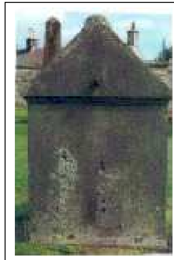
Figure 74 Moderate cratering and pitting
