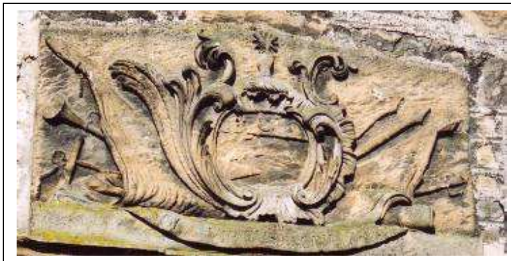
Figure 73 Minor surface loss
